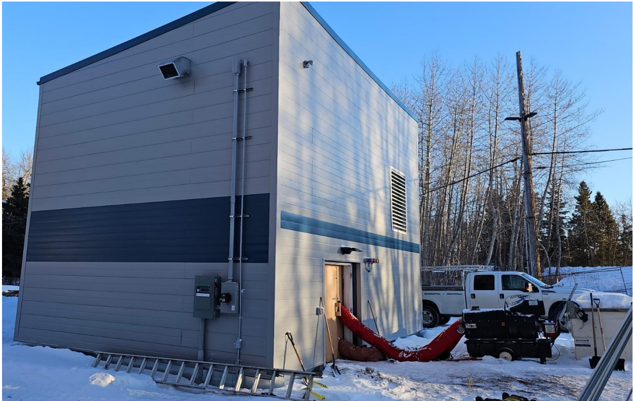
Hay River/Kát'odeeche – This Lift Station (currently under construction in the photo) has been wet-proofed and dry-proofed to withstand floods. All mechanical equipment is located on the second floor of the structure, and flood resistant materials are used throughout. (Photo courtesy of Glenn Smith)
