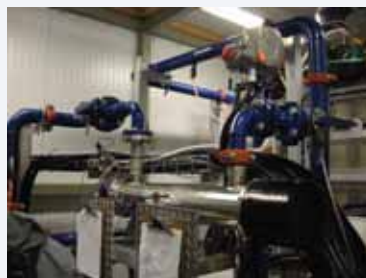
Ultraviolet Reactor: Ulukhaktok
