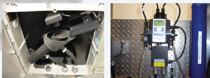
On-line Water Quality Testing Equipment (Left to Right) Turbidimeter - Service Scatter (measures high level turbidity) Ultraviolet Transmittance Meter
