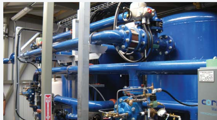
Pressure Filters in the Tuktoyaktuk Water Treatment Plant
