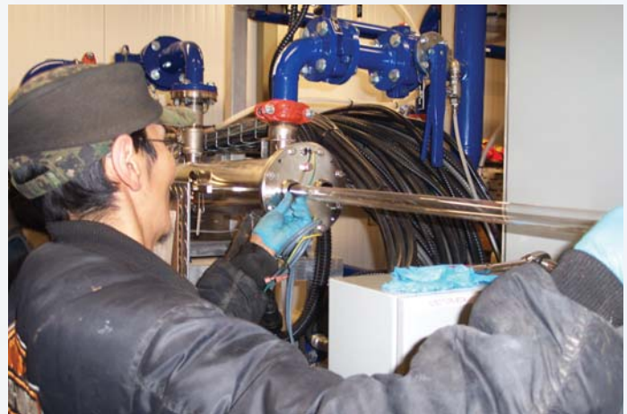
Ulukhaktok Water Treatment Plant Operator, Gibson Kudlak, Performing Maintenance Training on the UV System.
