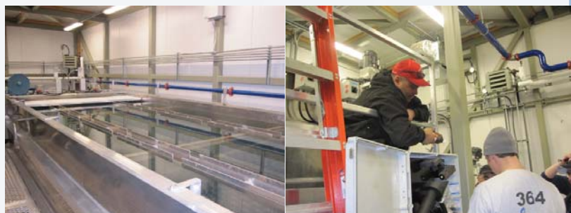
Aklavik Water Treatment Plant Treatment Train (Left), Operator Training (Right)
