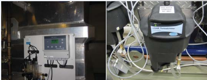
On-line Water Quality Analyzers for Remote Monitoring Chlorine (Left), Turbidity (Right)
